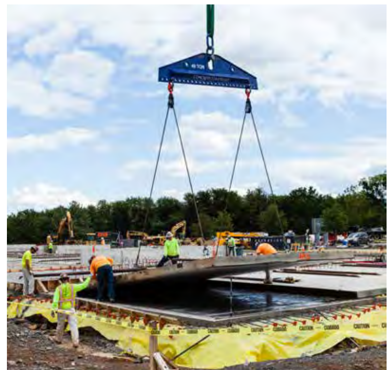
310 Innovation Boulevard featured an innovative build process called tilt-up construction that allowed for faster completion of the project.
